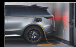
EV CHARGING POINT
